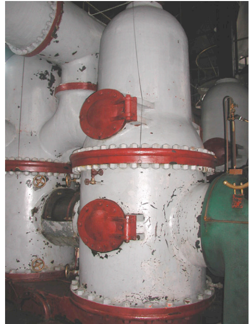
Figure F2. Worthington engine with CRC 3-36 corrosion suppressant coating.
