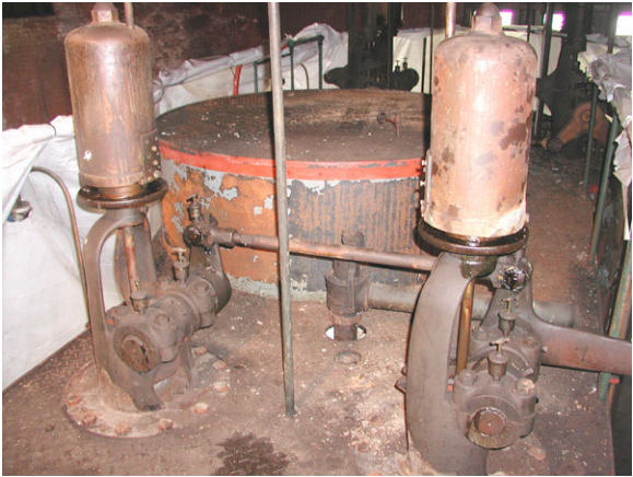
Allis Floor 4 mid detail C looking north before treatment.
