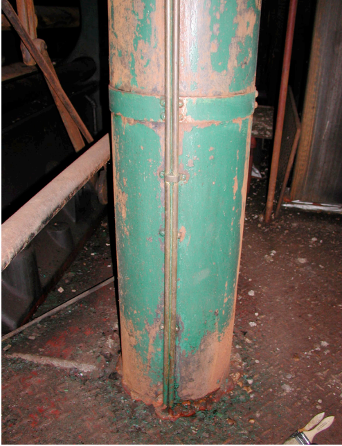
Figure B1. Originally painted surface, exhibiting extensive rust, Worthington engine before treatment.
