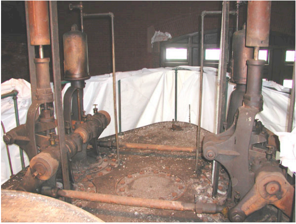
Allis Floor 4 North detail A before treatment.
