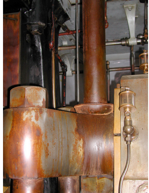
Figure A2. Rusted metal surfaces cleaned with mineral spirits and coated with Corrosion Suppressant 101- Allis engine after treatment.
