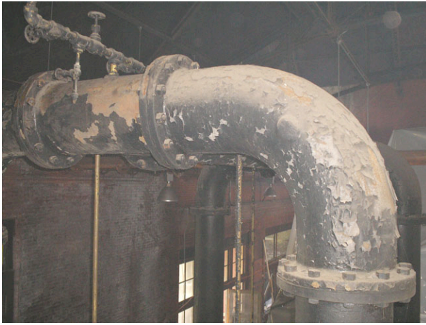
Worthington Floor 3 North detail A, before treatment.
