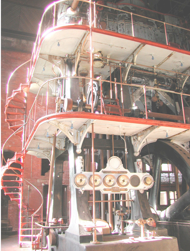
Allis engine (southeast elevation) before Treatment November 21, 2005.
