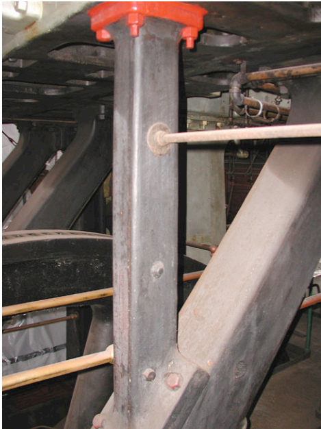
Leavitt Floor 2 North end detail E, north side before treatment.
