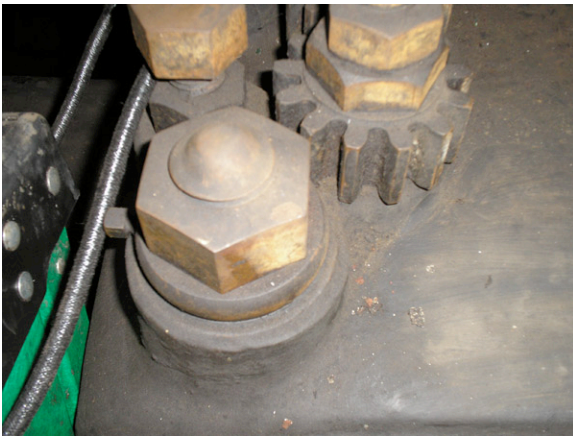
Figure I1. Leavitt engine, first floor bolt, detail before cleaning.
