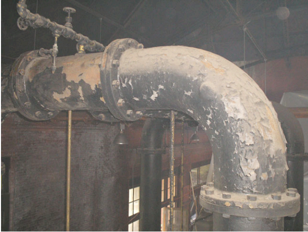
Worthington Floor 3 North detail A, before treatment.
