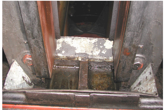
Figure K2. Standing oil build-up at Allis engine after treatment.
