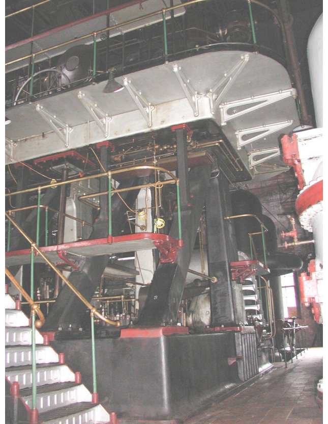
Leavitt engine (northwest) after treatment August 30, 2006.
