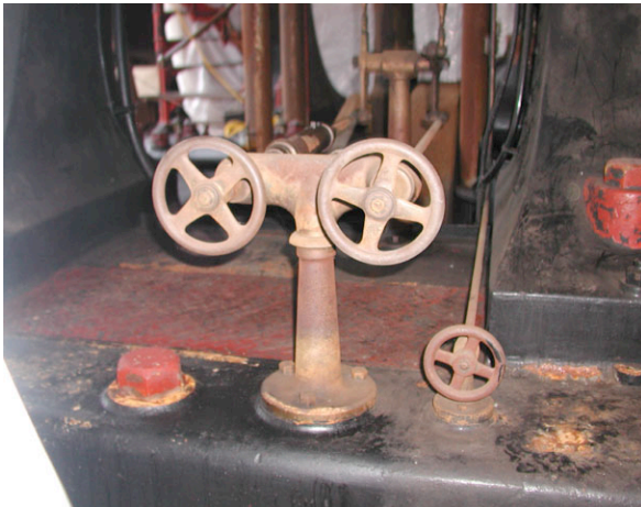
Allis Floor 1 South detail G, east side before treatment.
