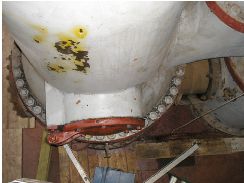
Figure F1. Worthington engine north end with CS 101 corrosion suppressant coating.
